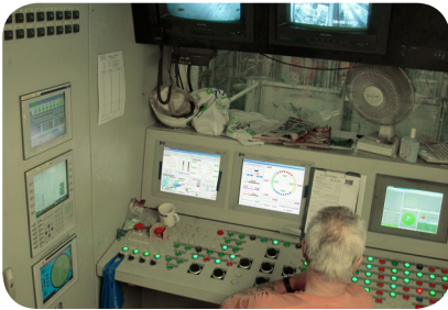
Kommandoraum TBM Control room of TBM
